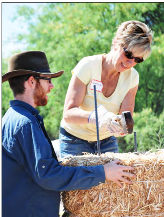
Volunteers build a straw bale wall at the entrance to Feld Davis Park.
