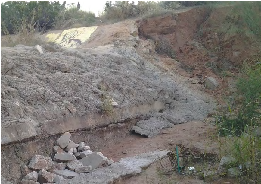
Figure 3 - - Grade control structure directly downstream of Transect 2. Note destructive erosion of west wing wall.
