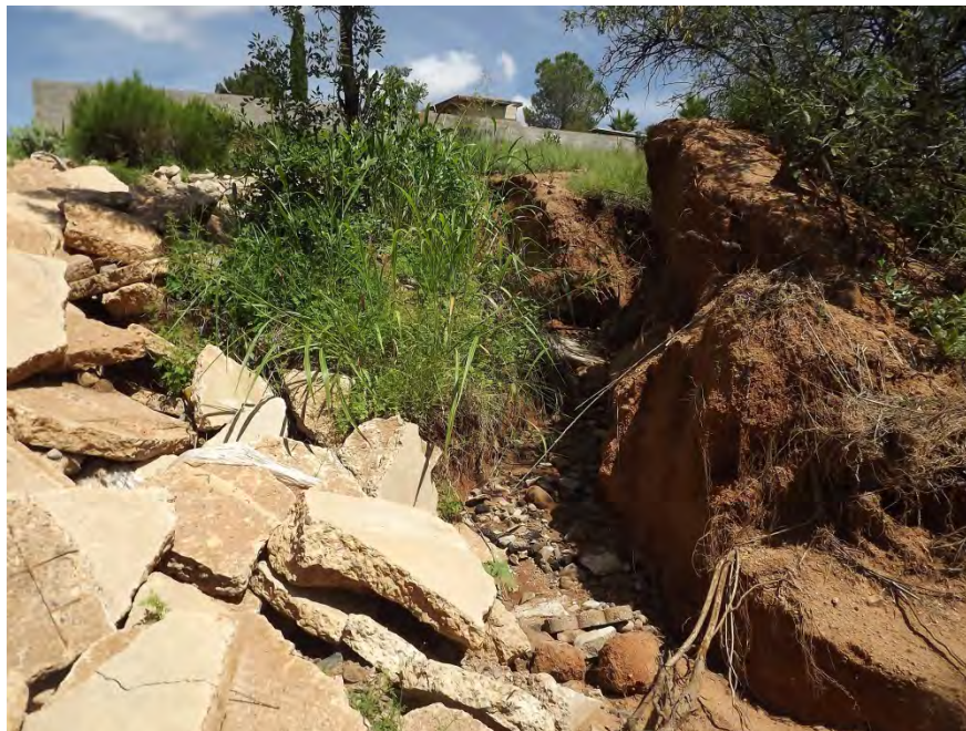
Figure 4 - - Carmelita Avenue outfall looking north from channel grade. Severe erosion is obvious.
