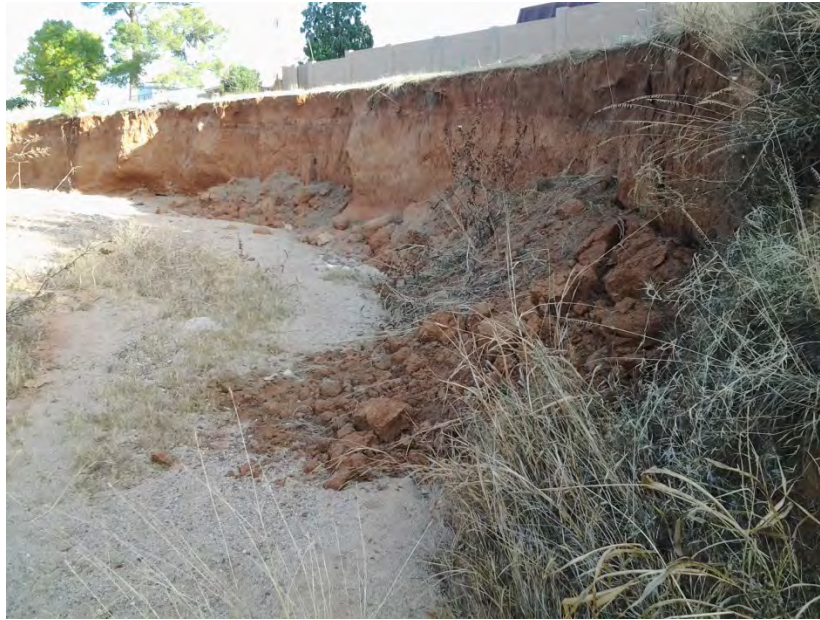
Figure 5 - - Approximately three-meter high cut bank on the southeast bank of Buena #3. Basal debris in center from a failure recent enough to expose roots of still living grasses.
